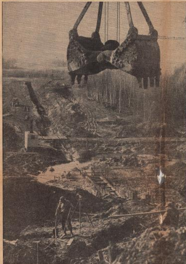
DAM FOR COLONIE WATER SUPPLY BEING BUILT ACROSS STONY CREEK IN THE TOWN OF CLIFTON PARK
